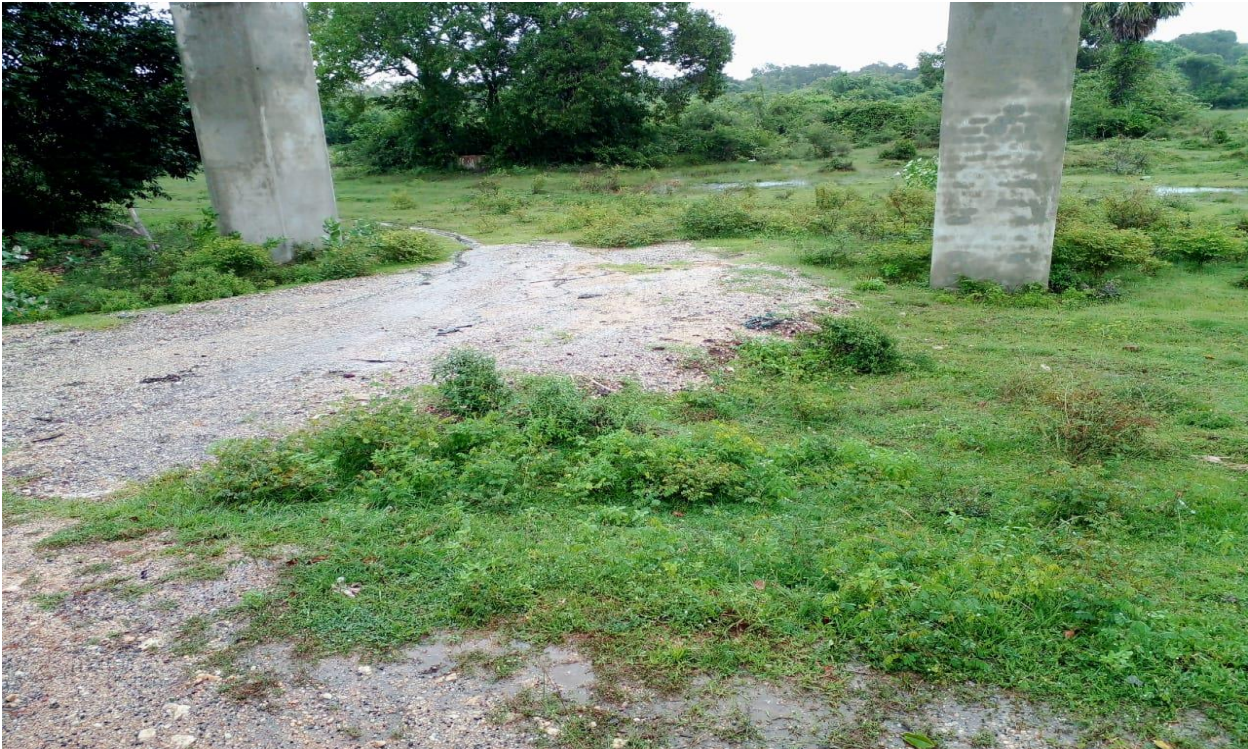
The access road being constructed by the National Youth Service Council through the authority's land
