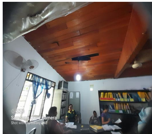
Non-maintenance of buildings Galgamuwa Samurdhi Bank- 16 May 2023
