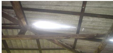
Damaged roof in Masonry Section at the MCS
