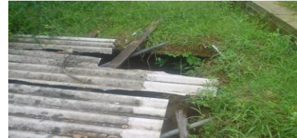
Unprotected Toilet Pit at Makola Certified School
