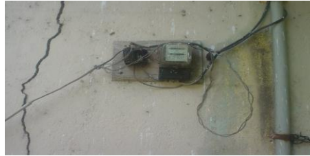
Unsecured Electricity System at the RRH
