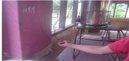
Unsecured Electricity System at Makola Certified School
